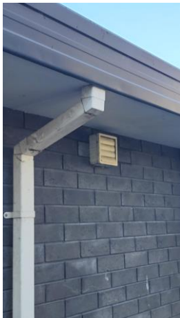
Kitchen ext vent
