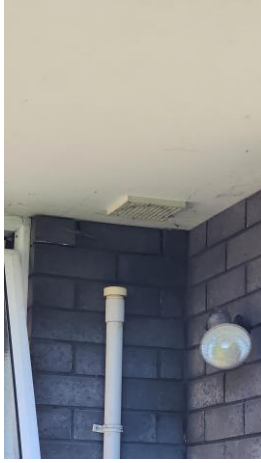
Bathroom 2 Ext Vent
