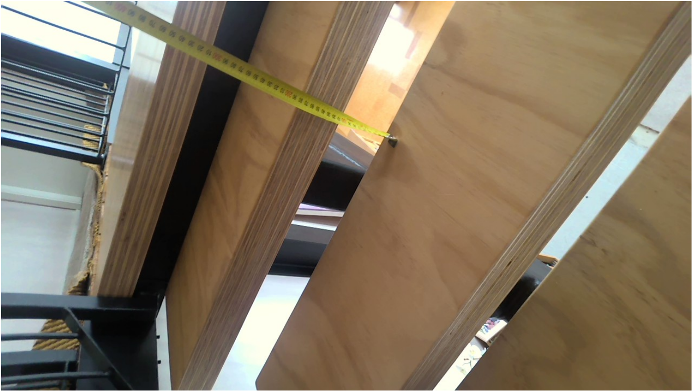
Not uniform with rest of stairs Taken at 9:17 AM on Thursday 28/11/2024
