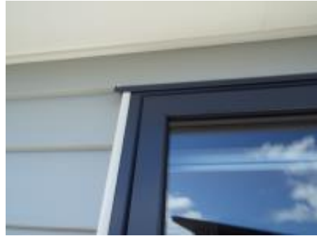
good flashing detail
