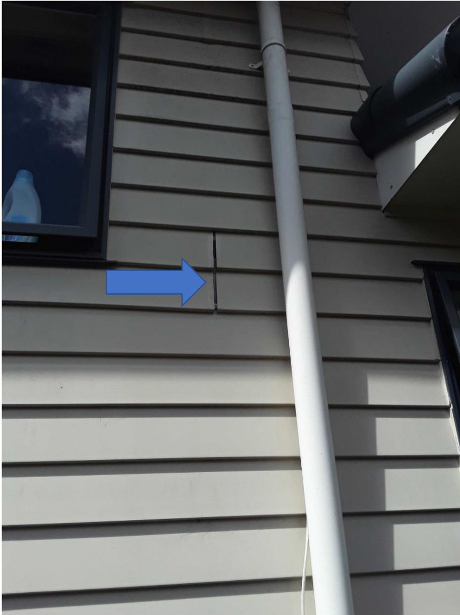
Blue arrow – Missing jointer
