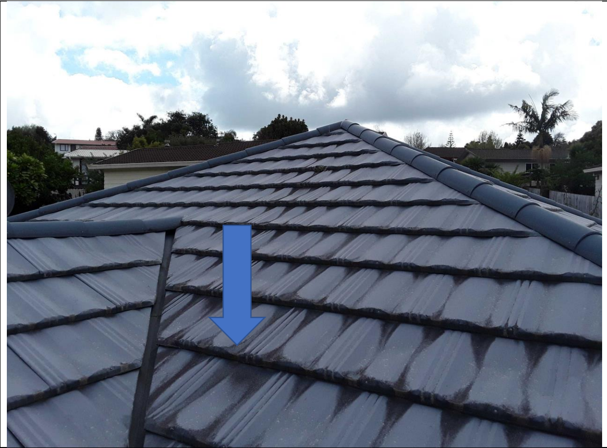
Blue arrow – Dirty with moss and mould growing, needs a clean
