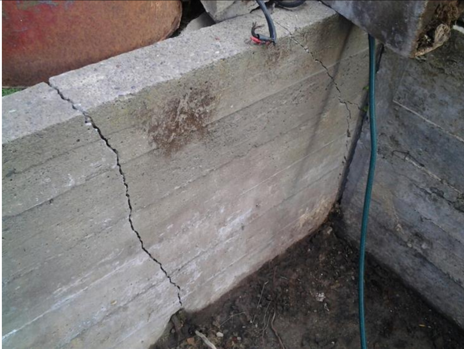
Vertical cracking to the far RHS of wall 6
