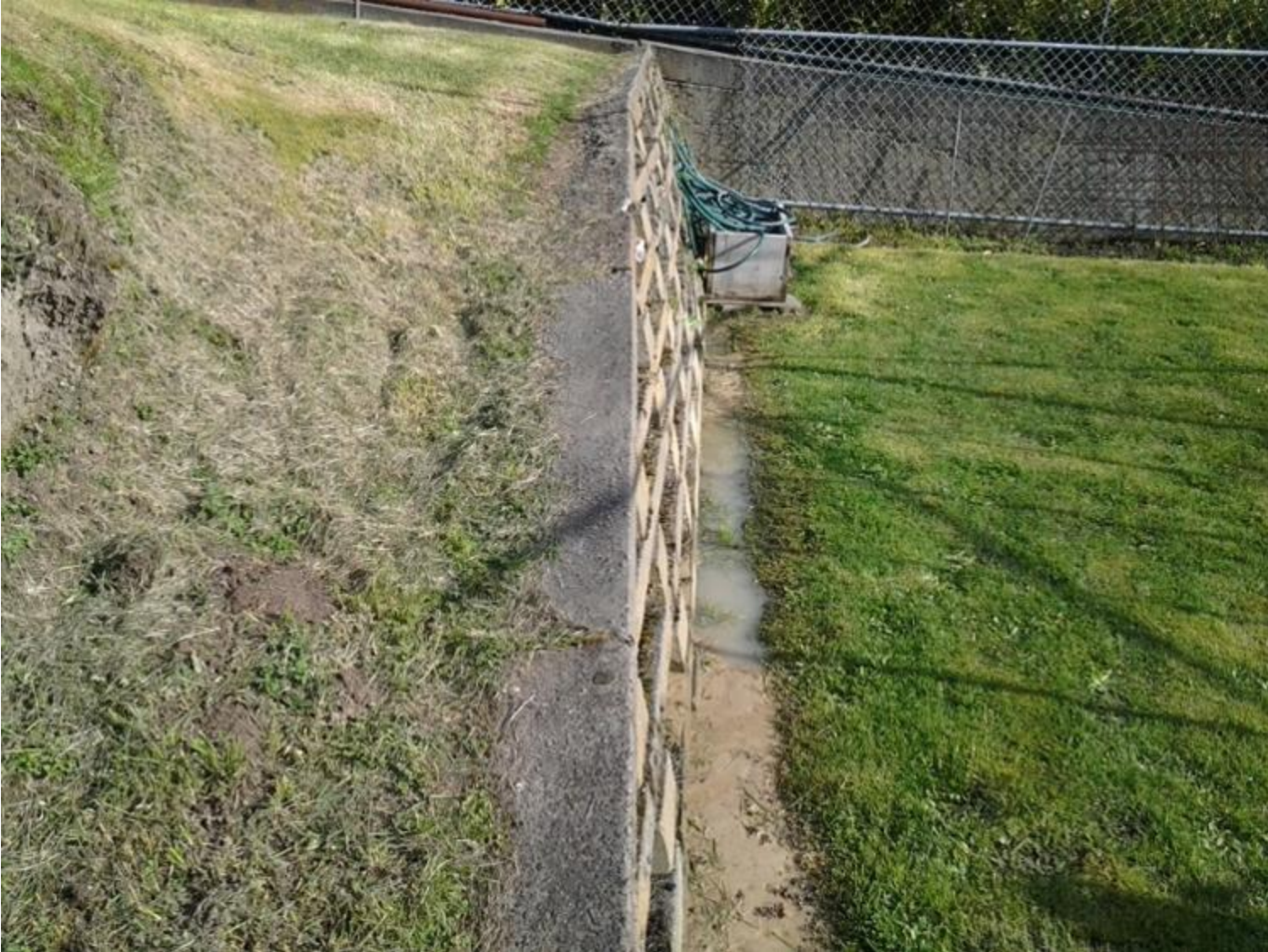
Misalignment to the cribs within the wall
