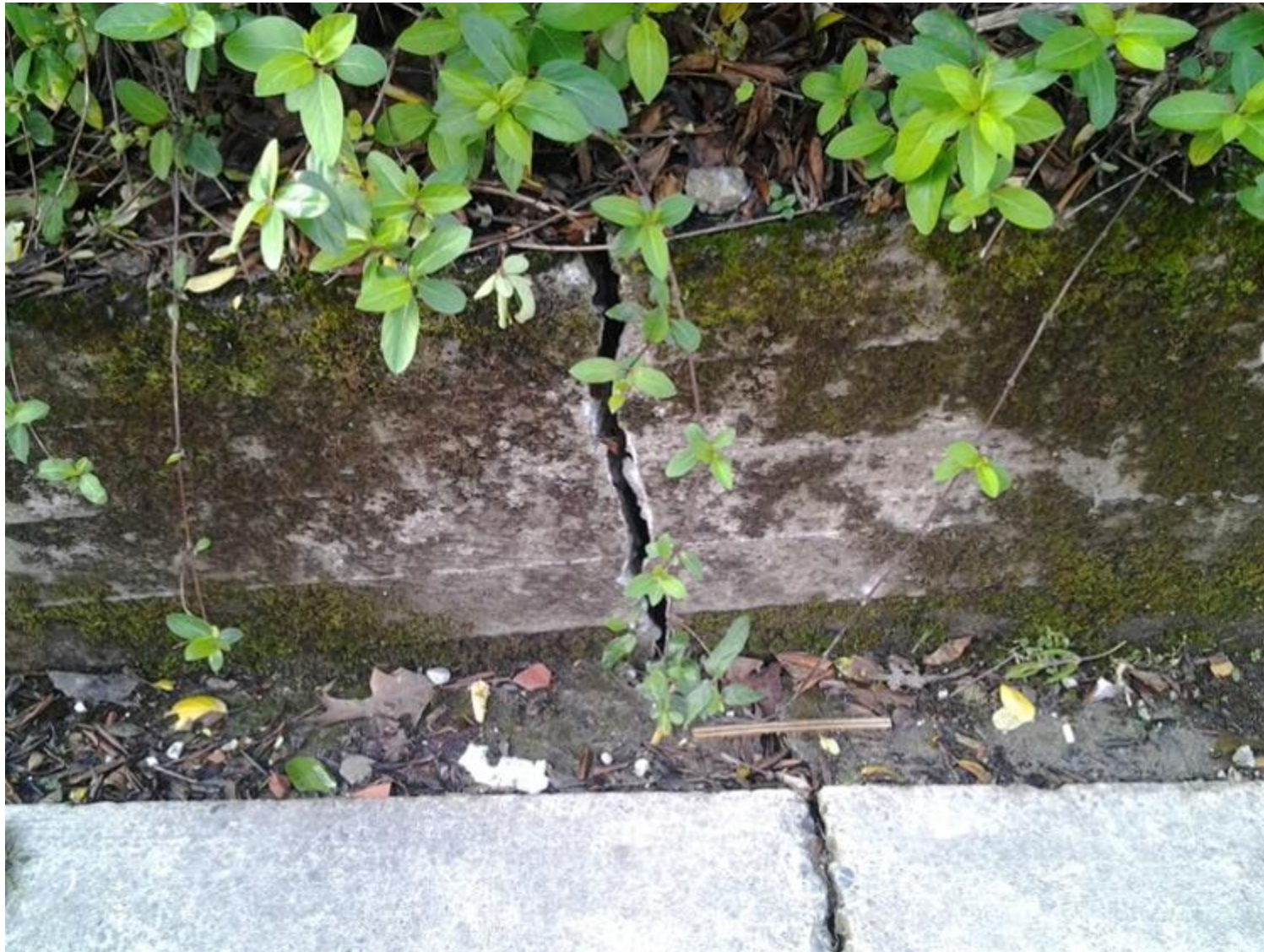
Vertical cracking to wall 4
