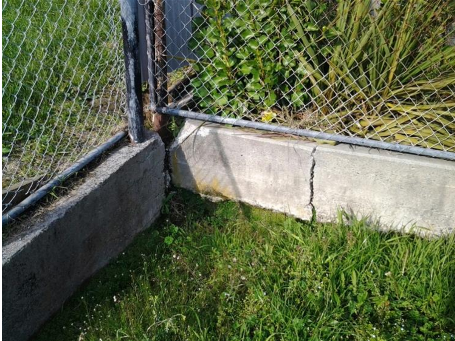
Cracking to wall 5 in the top LHS corner of the section
