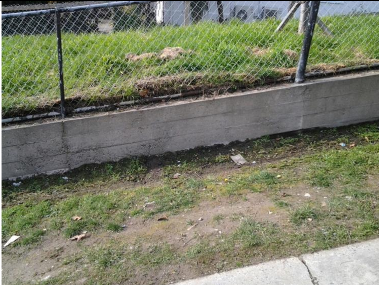
Vertical cracking to LHS of wall 5
