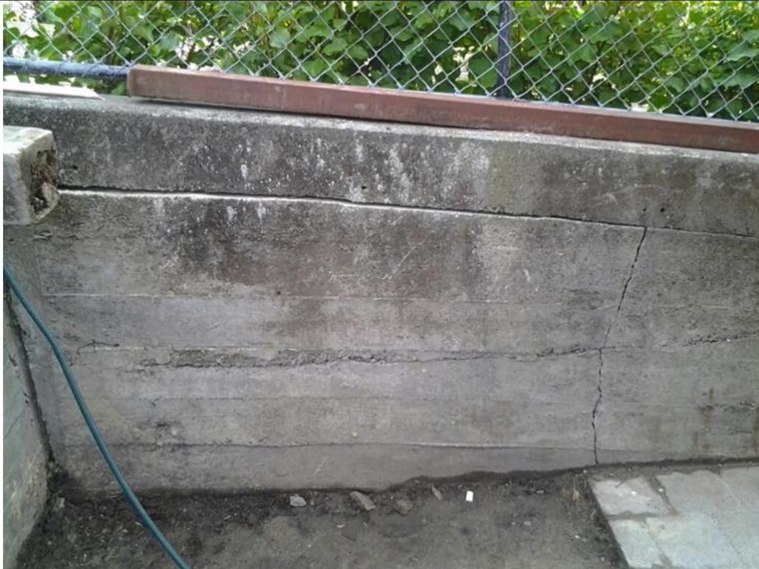
Vertical and horizontal cracking to the RHS of wall 5 behind the house
