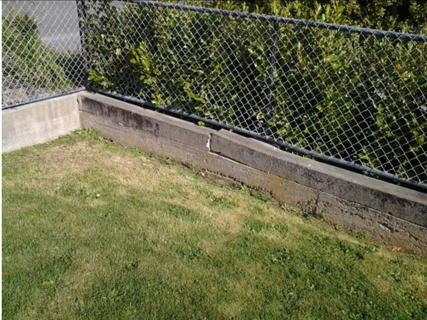
Cracking to wall 5 in the top RHS corner of the section
