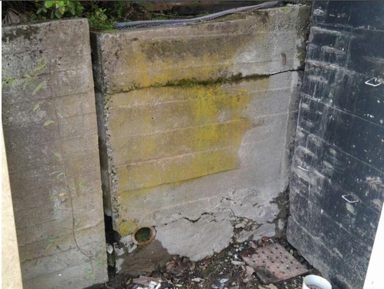
Seperation and horizontal cracking to wall 4 in front of the garage
