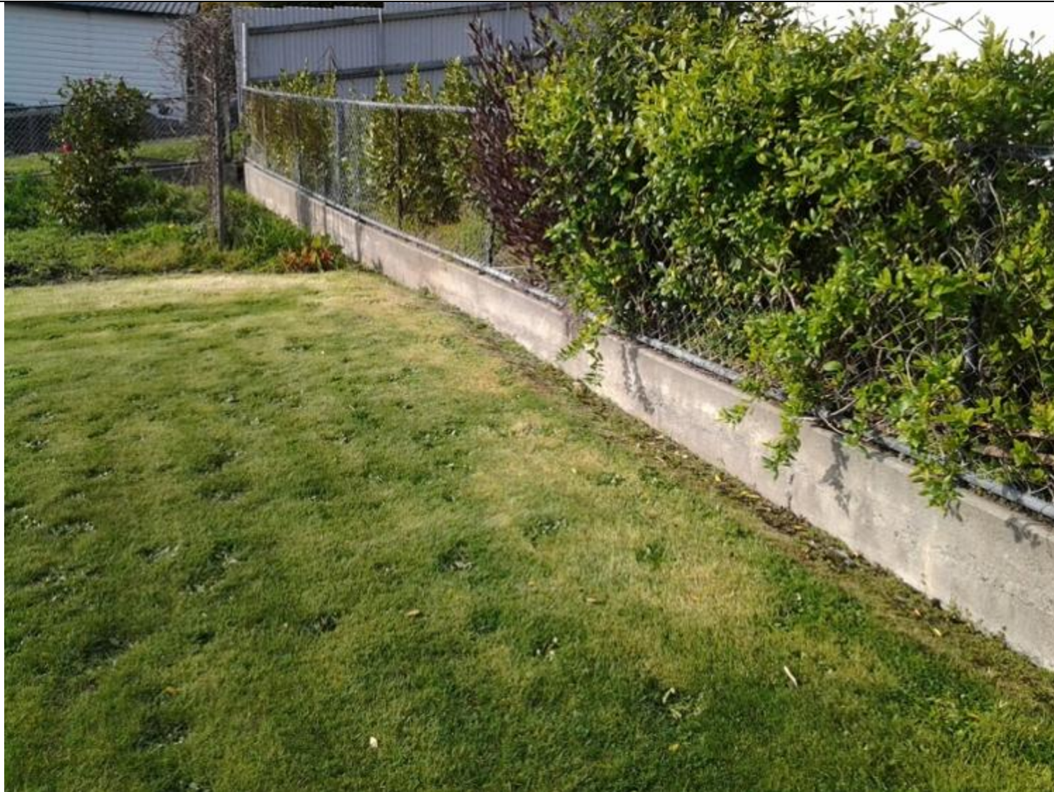
Elevation of wall 5 across the rear of the section from the RHS
