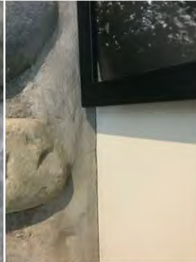
5. Entry (1.00) movement between stone and wall, minor cracking to mortar
