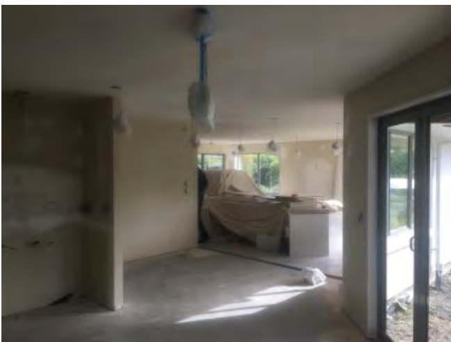
Kitchen - Plasterboard lining repairs complete, painting underway, cabinetry and bamboo flooring removed
