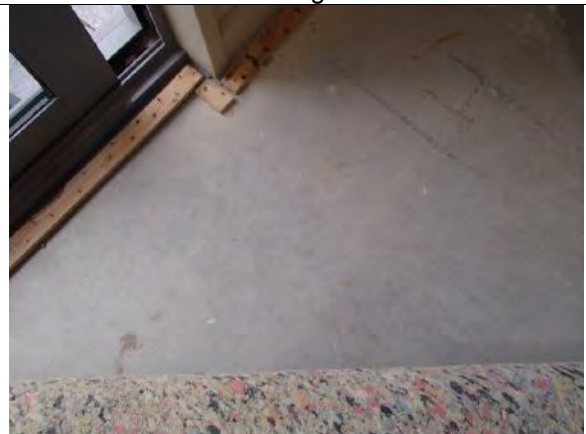
Photo 16: Image provided by the homeowner of cracking within the bedroom 4 (room 1.13) concrete slab-on-grade
