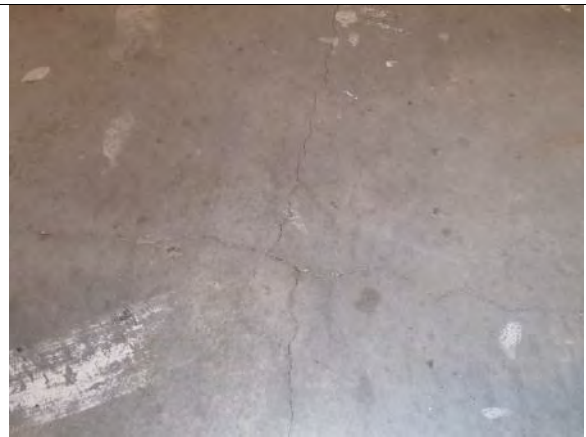
Photo 14: Image provided by the homeowner of cracking within the lounge (room 1.05) concrete slab-on-grade
