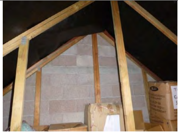
Photo 20: View of the masonry firewall located between the managers' residence garage (room 1.17) and the adjacent apartment wing
