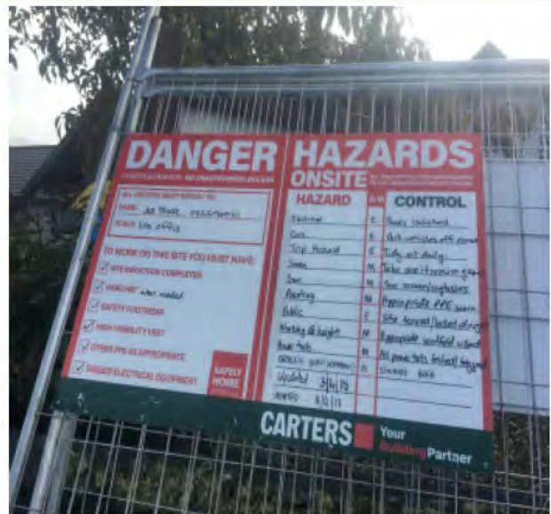
Up to date Hazard Board
