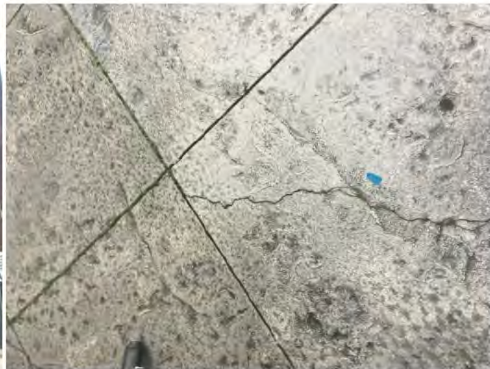
11. Typical cracking of cut concrete patios
