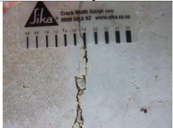
Photo 12: Cracking within the garage approximately 1.8 mm in width
