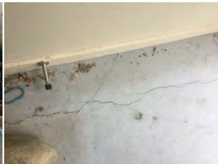
14. Garage (1.17) cracking to slab
