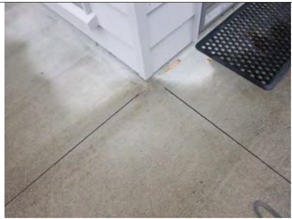
Photo 8: Cracking in adjacent external paved surfaces
