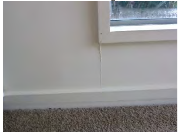
Photo 18: Typical cracking within the managers' residence plasterboard linings
