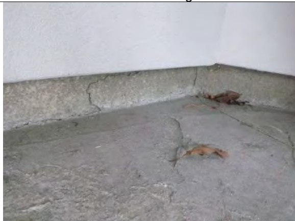
Photo 17: Perceived cracking in the side of the managers' residence slab-on-grade; however, this is likely to be screed remnants from the adjacent external concrete surface
