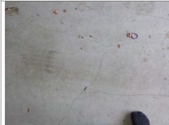
Photo 9: Typical cracking within the garage concrete slab-on-grade
