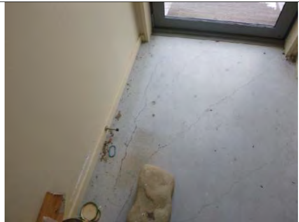
Photo 10: Cracking within the garage concrete slab-on-grade
