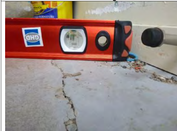
Photo 11: Variation in floor level adjacent to cracking within the garage
