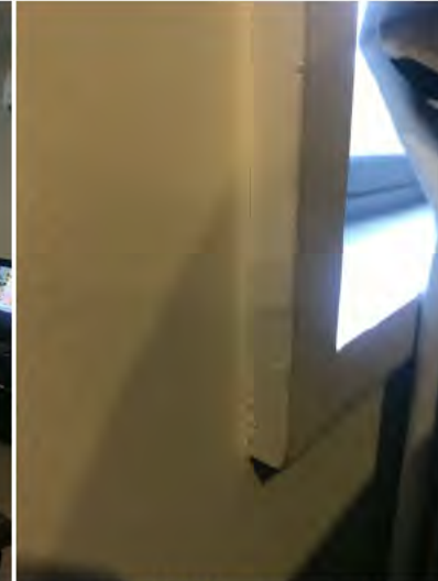
8. Family (1.01) movement to window and wall cracking
