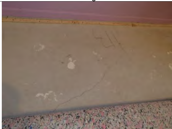
Photo 15: Image provided by the homeowner of cracking within the bedroom 2 (room 1.10) concrete slab-on-grade
