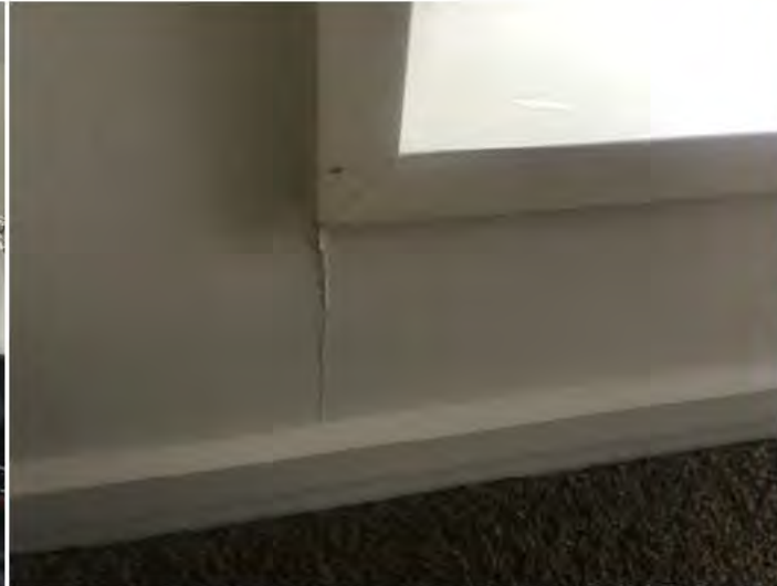
2. Lounge (1.05) cracking under window
