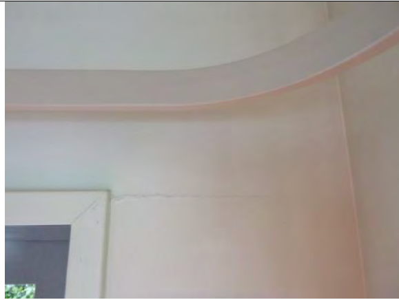
Photo 19: Typical cracking within the managers' residence plasterboard linings
