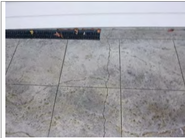
Photo 7: Cracking in adjacent external paved surfaces
