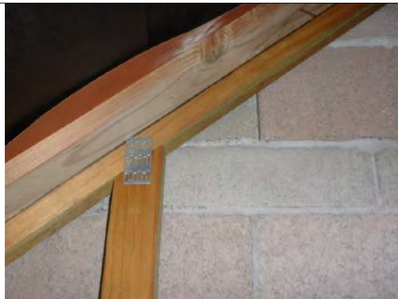
Photo 21: Perceived dislocation within the firewall between the managers' residence garage (room 1.17) and the adjacent apartment wing
