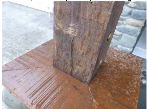
Photo 22: Split within a timber post supporting the canopy extending beyond the garage (room 1.17)
