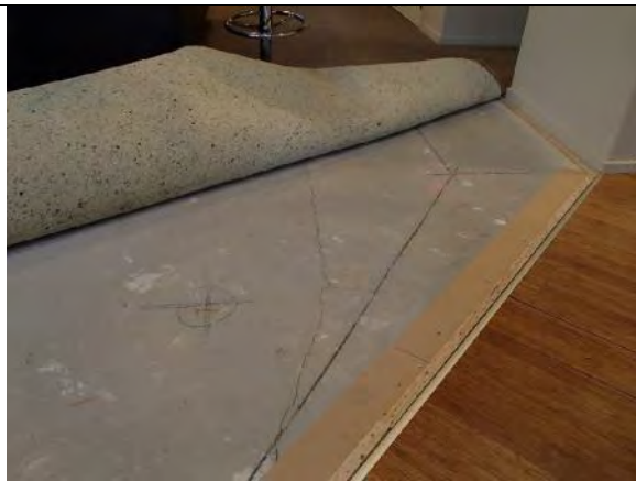
Photo 13: Image provided by the homeowner of cracking within the kitchen (room 1.02) concrete slab-on-grade
