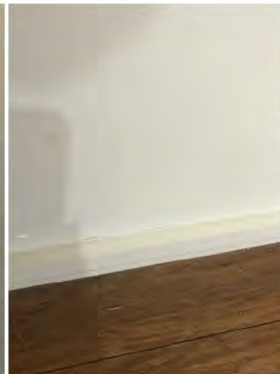
14. Kitchen (1.02) movement to skirting
