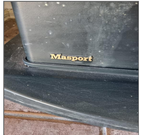
Heating - Pre-existing heater
