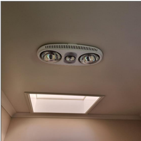
Bathroom 1 Ventilation (Extraction Fan) - Fan in good working order
