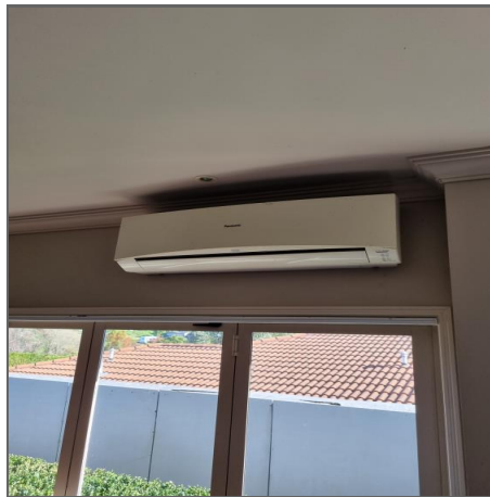
Heating - Pre-existing heater
