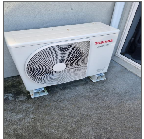
Heating - Pre-existing heater
