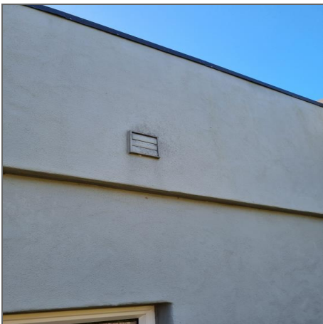
Bathroom 2 Ventilation (Extraction Fan) - Additional photo
