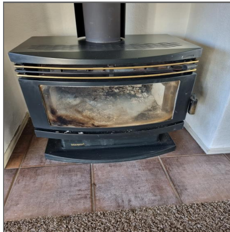
Heating - Pre-existing heater
