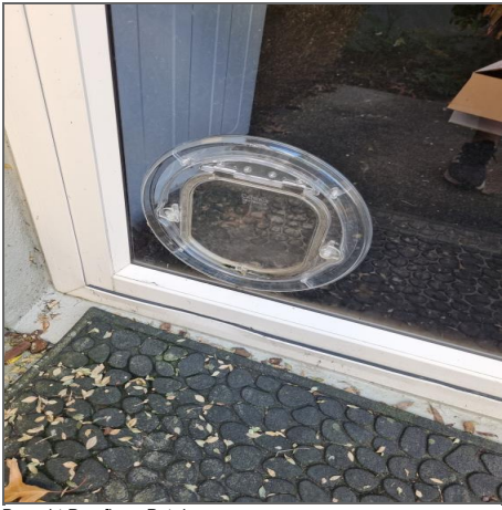
Draught Proofing - Pet doors gaps
