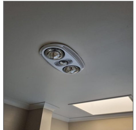
Bathroom 2 Ventilation (Extraction Fan) - Fan in good working order
