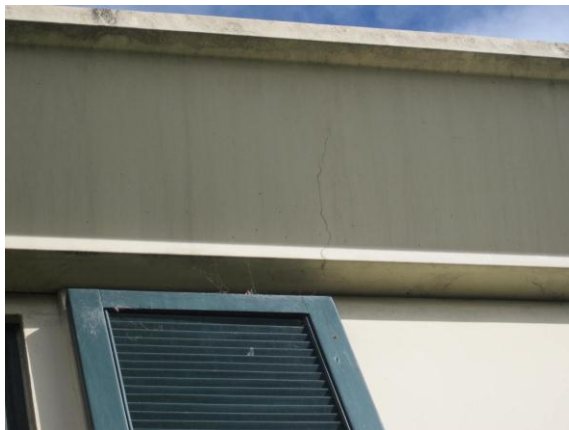
Crack at parapet, front elevation
