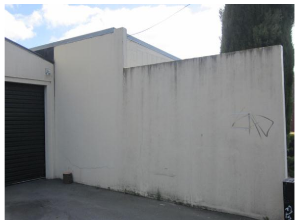
Cracks in adjacent wall along boundary
