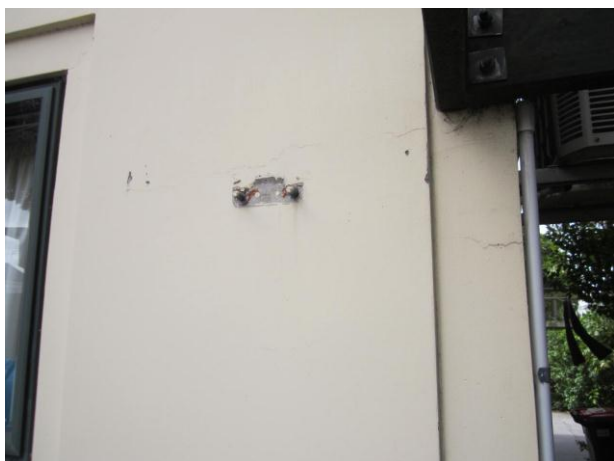
Crack at rear corner, ground floor
