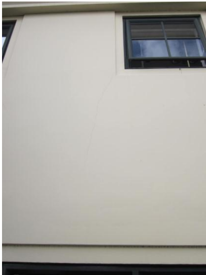
Crack near rear window, first floor
