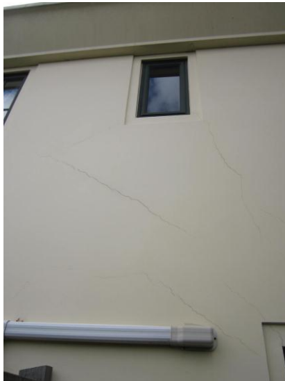
Crack at rear wall, first floor
