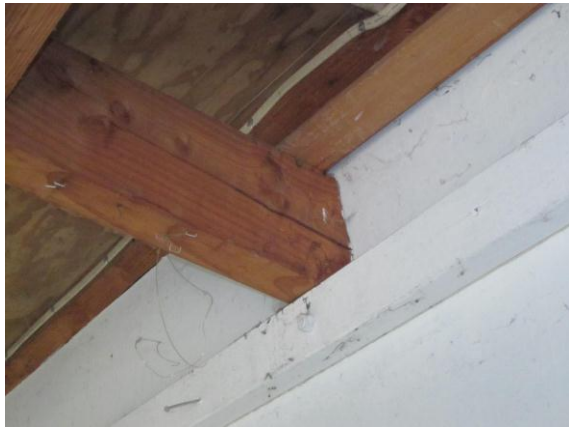
Lean-to roof joist splitting
