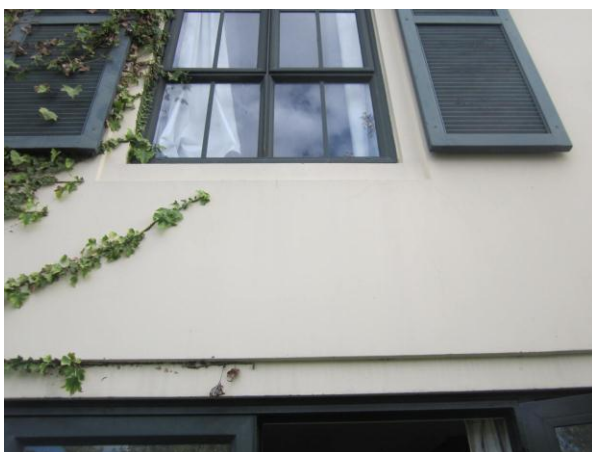
Crack above entrance
