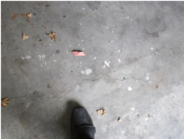
Crack in garage slab
