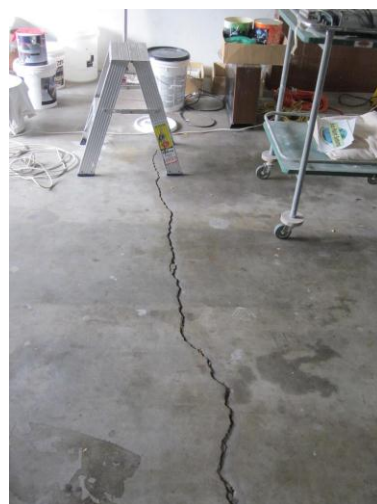
Crack at garage slab
