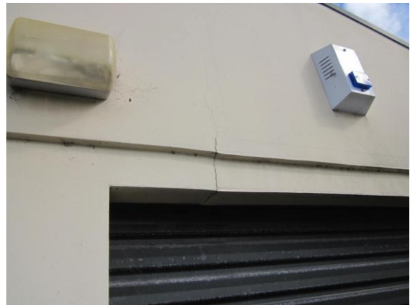
Crack at garage door lintel
