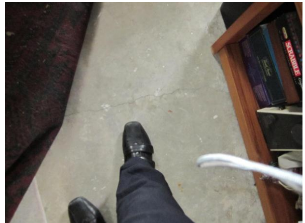
Crack in living room slab
