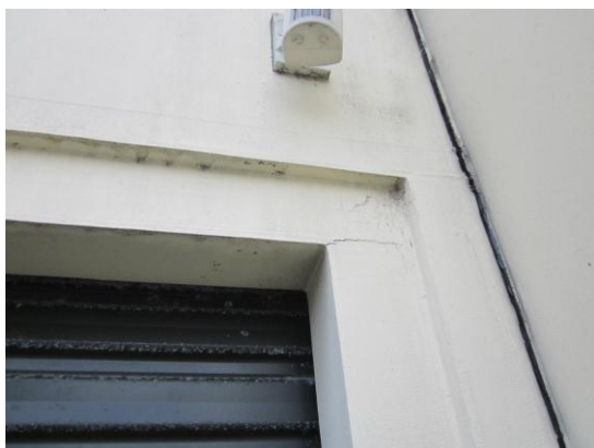
Crack at garage door, separation to adjacent wall
