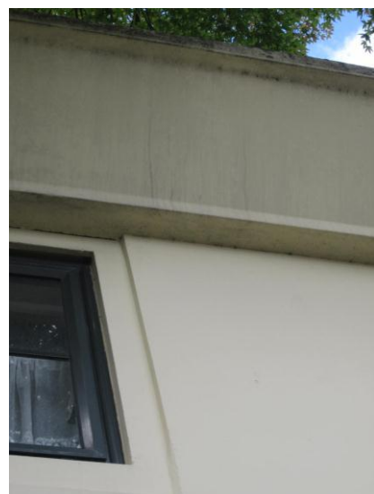
Crack at parapet
