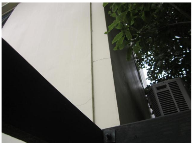
Crack at rear corner, ground floor
