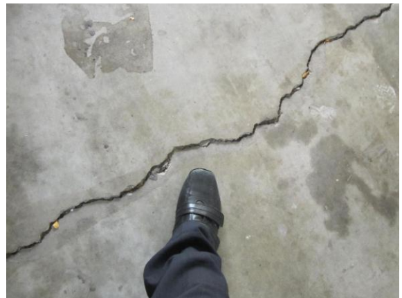
Crack at garage slab
