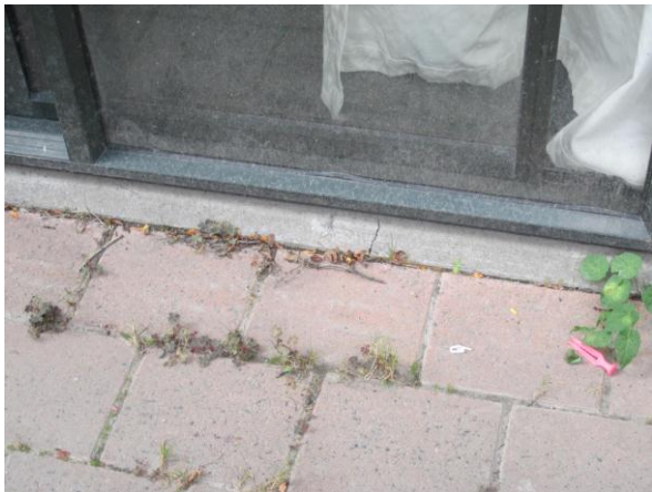
Crack at slab edge, entrance
