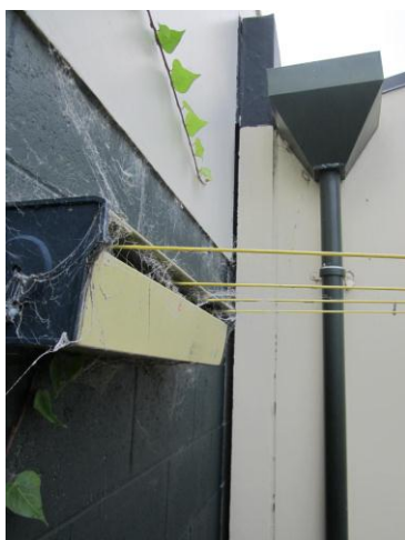
Separation at rear of garage
