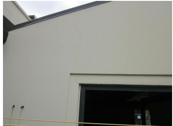
Crack at rear garage wall
