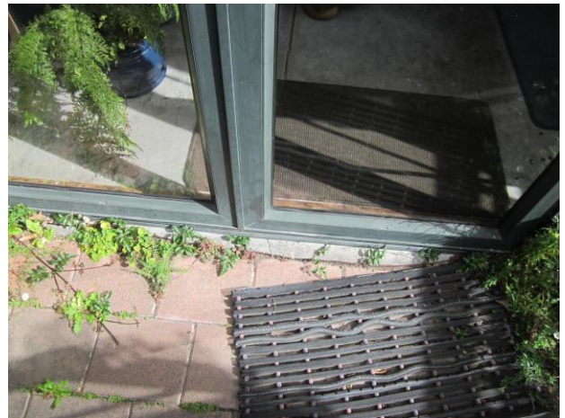
Crack at slab edge, entrance
