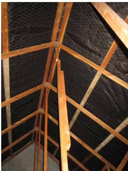
Disconnected roof tie
