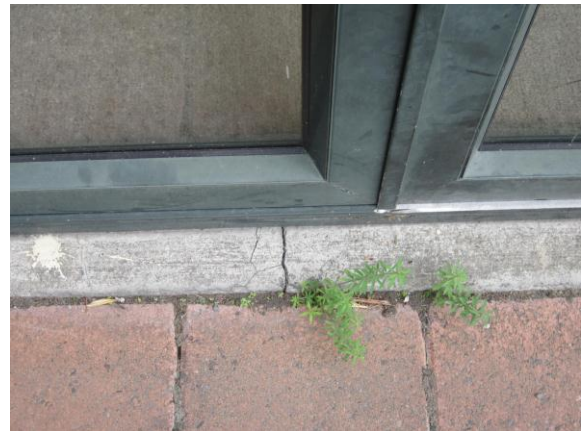
Crack at slab edge, front entrance
